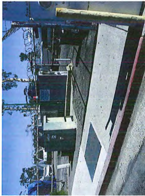
VIEW 9 - SEWER LIFT STATION NO. 11
